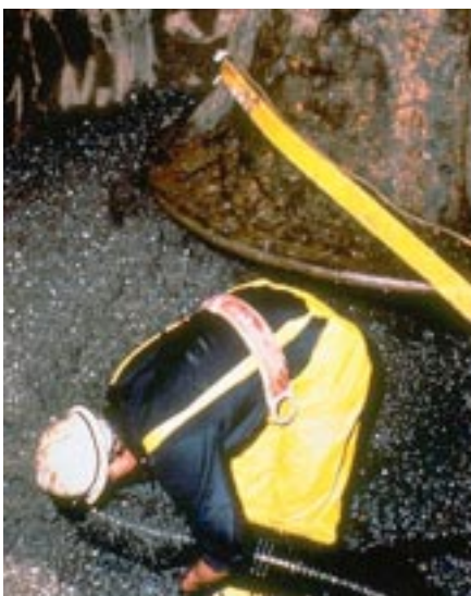
Worker removing zebra mussels from water intake pipes. Photo: Ron Peplowski, Detroit Edison—Monroe, Michigan Power Station
